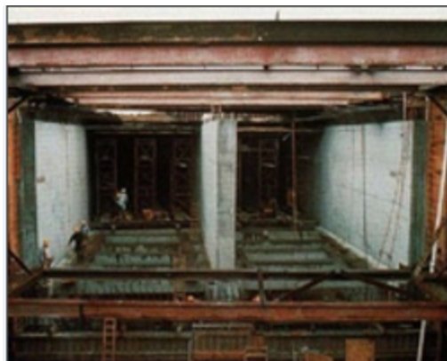
Construction of the Bayside and Westside Wet Weather Facilities was completed in 1997.
